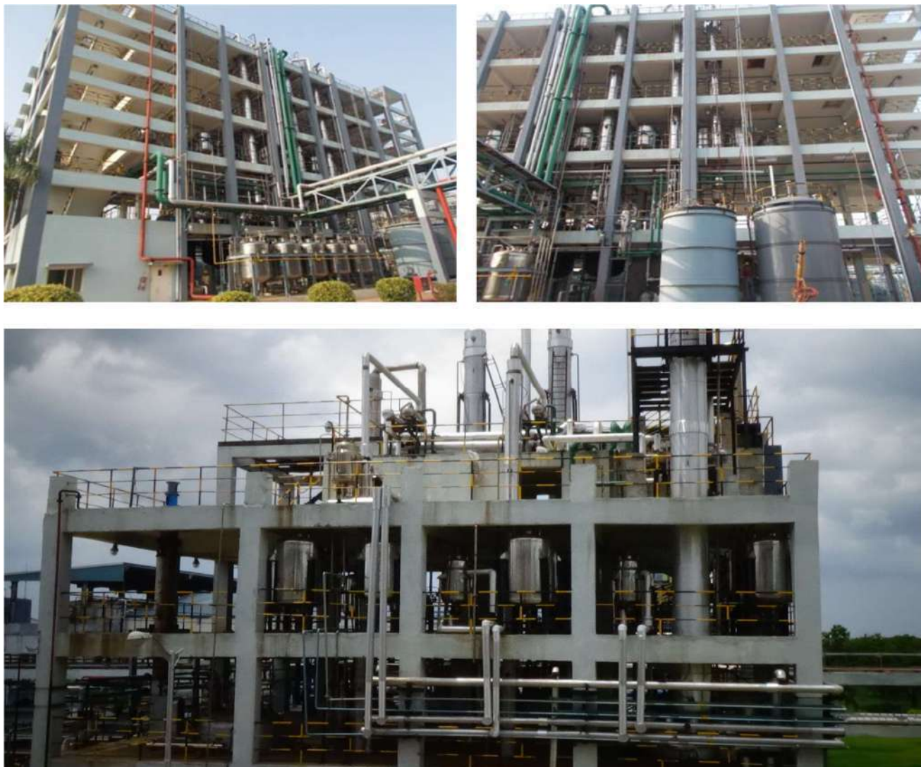
Fig 10.4 Photographs of existing Solvent Recovery System
