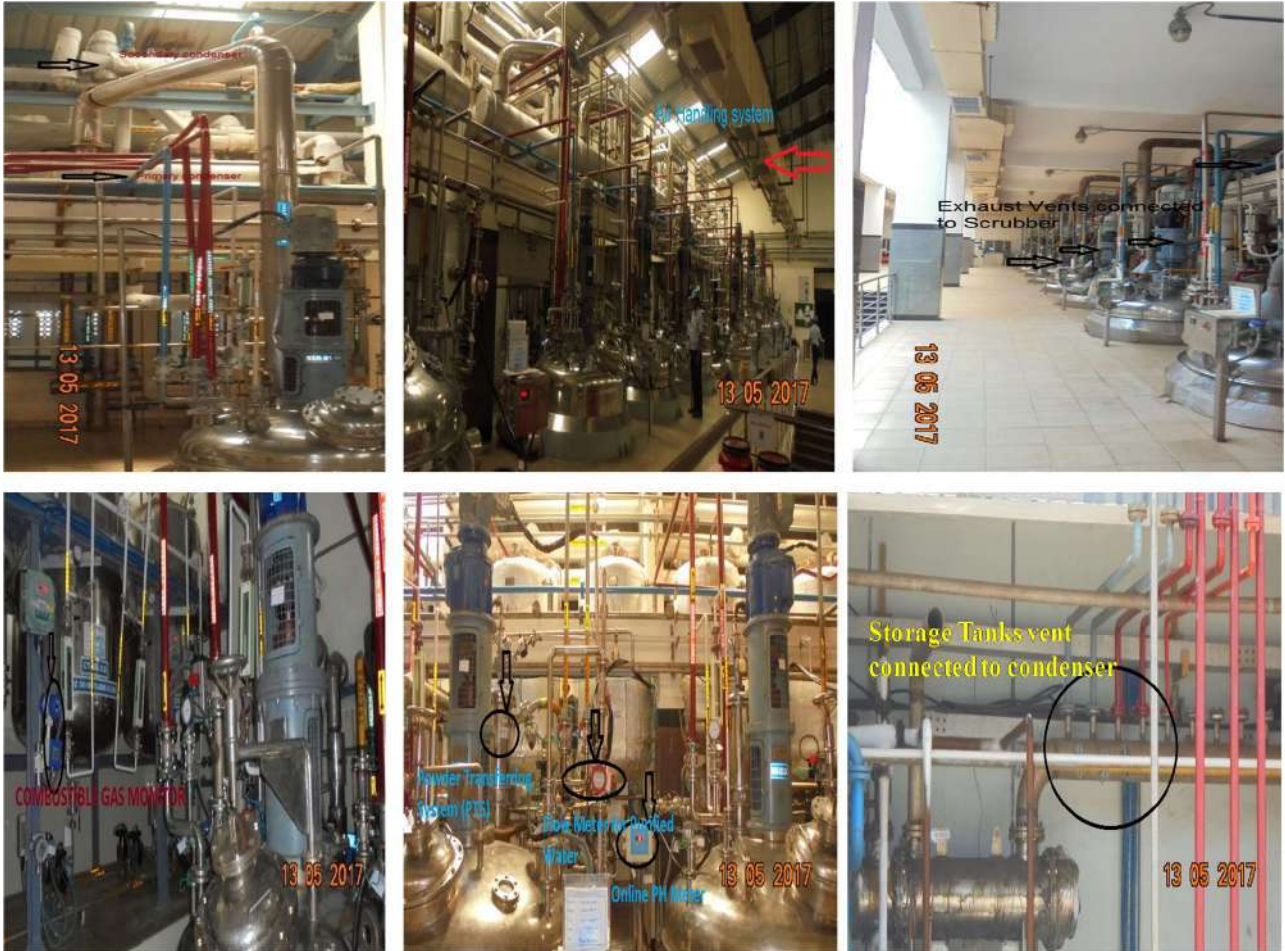
Existing Engineering Controls to Mitigate Diffuse and Fugitive Losses
