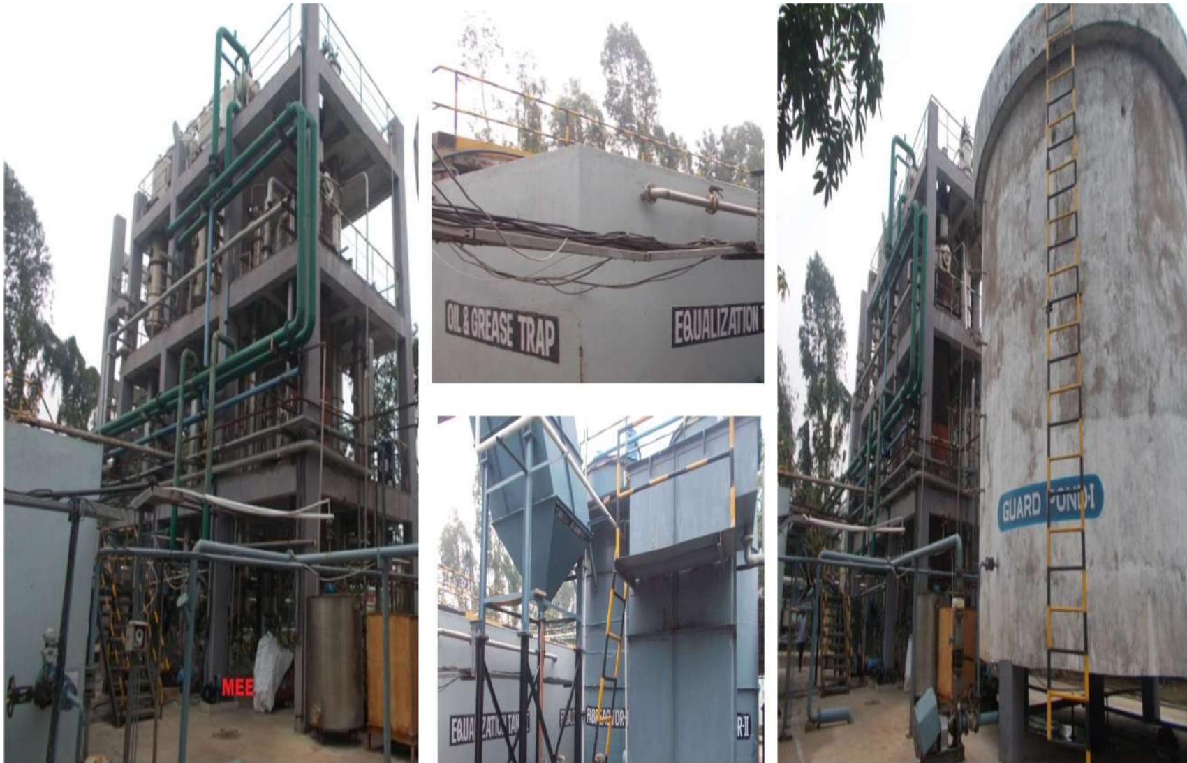
Existing Treatment System - Photographs
