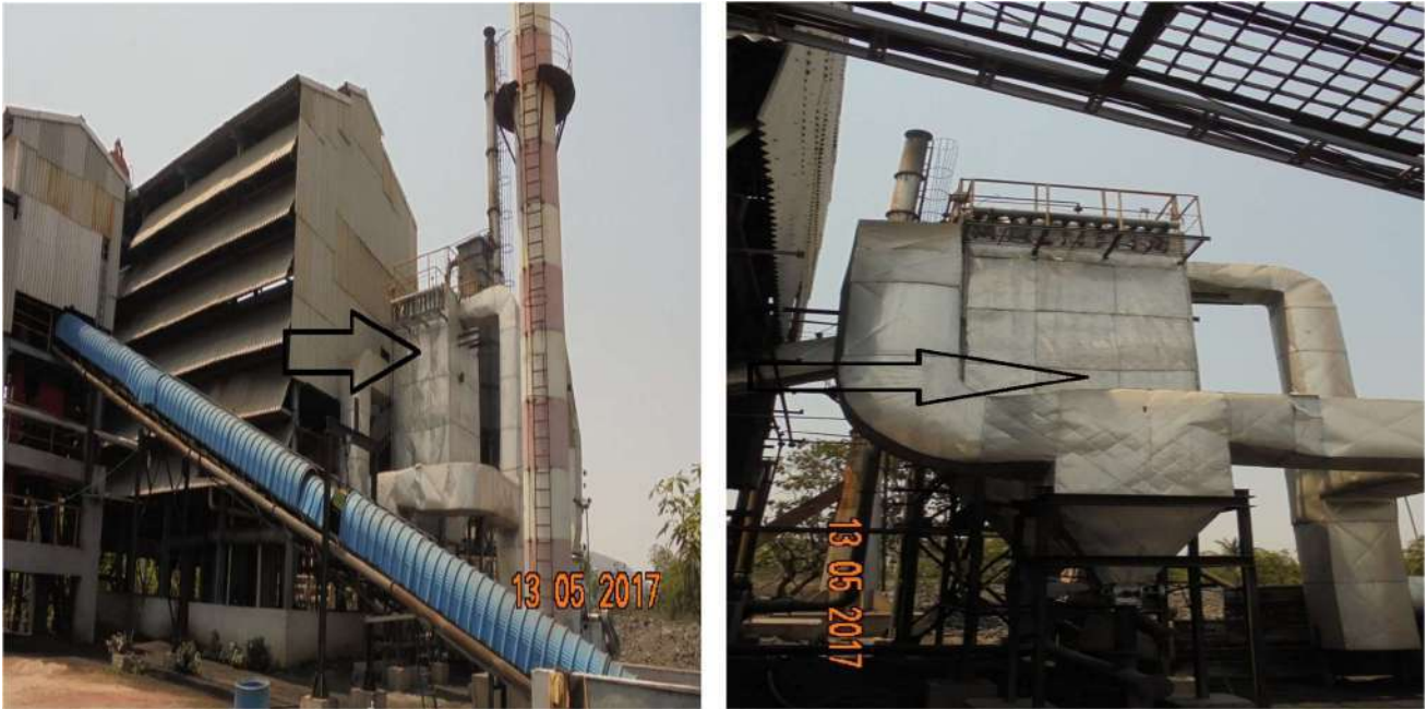
Photographs of Existing Boilers Stack connected to Bag Filters
