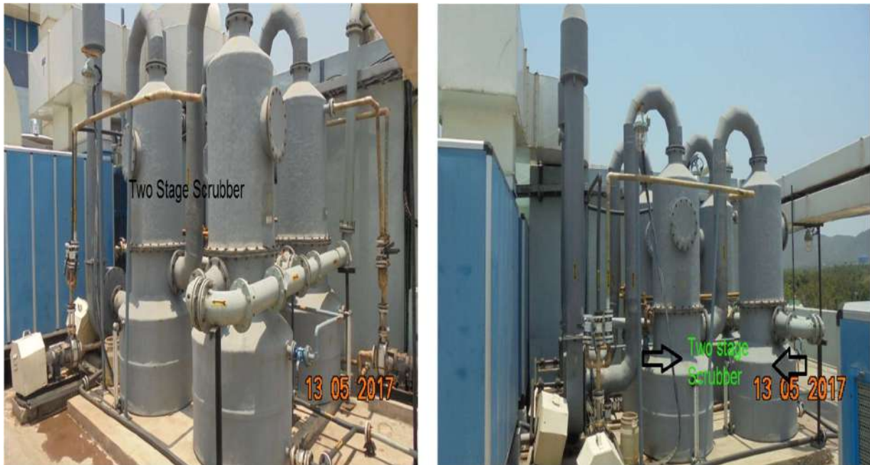
Fig 2.2 Existing Two Stage Scrubbing System
