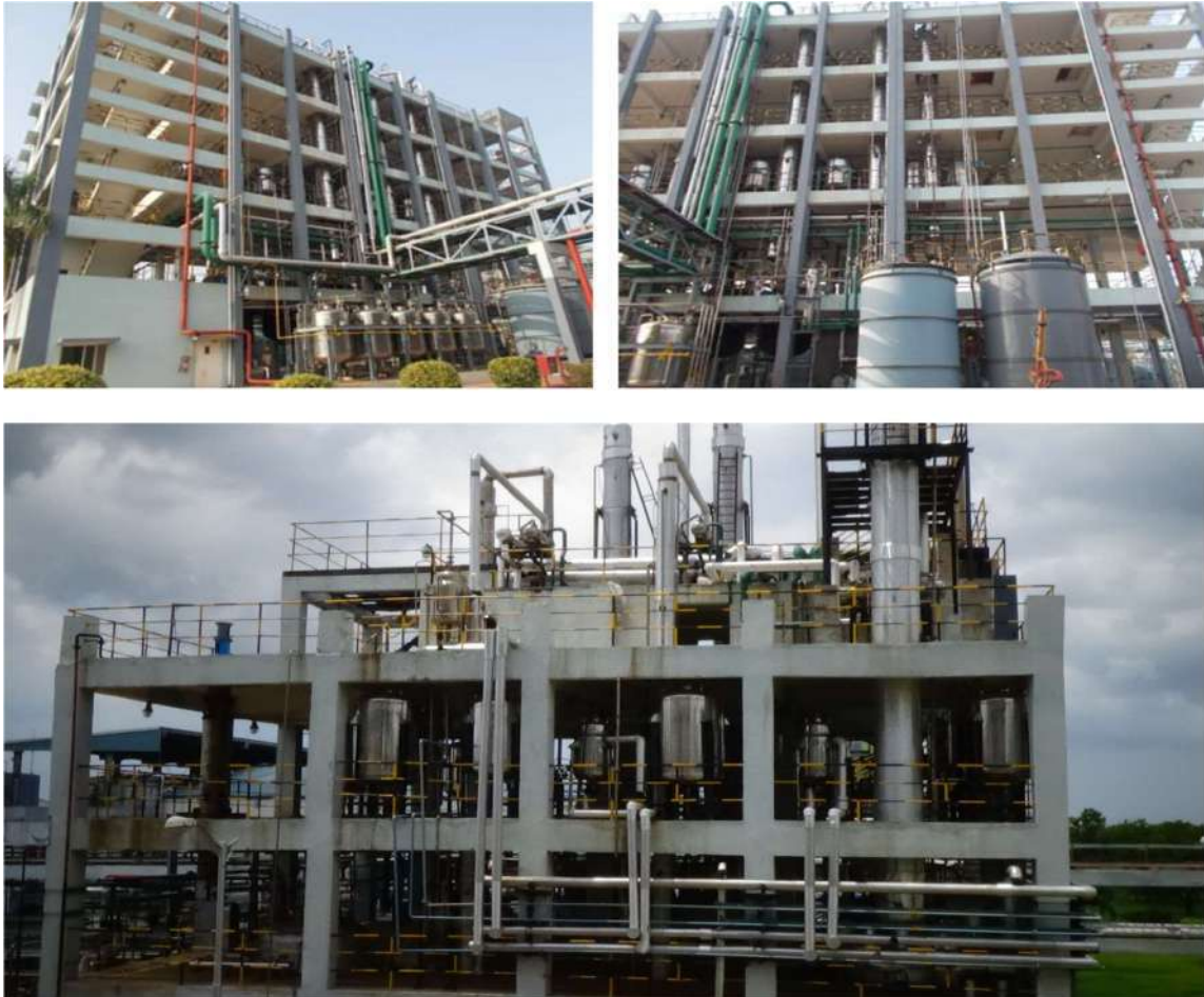
Fig 2.3 Photographs of existing Solvent Recovery System
