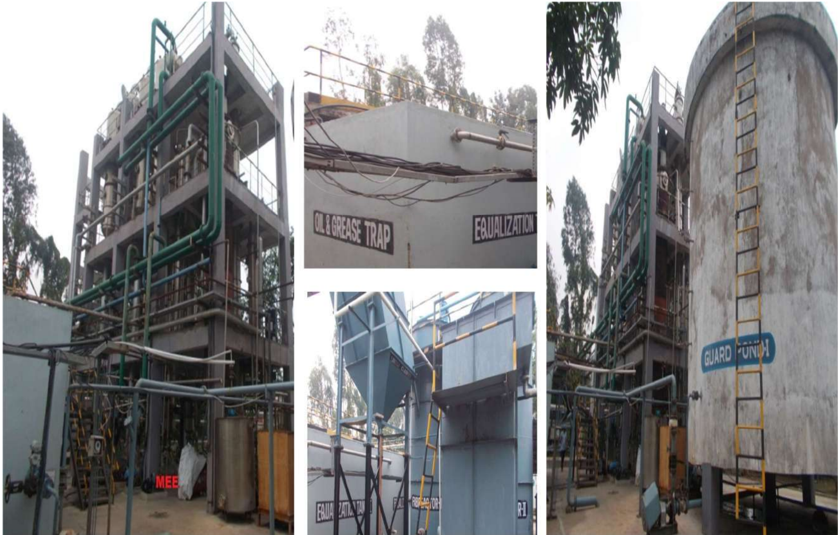
Existing Treatment System - Photographs
